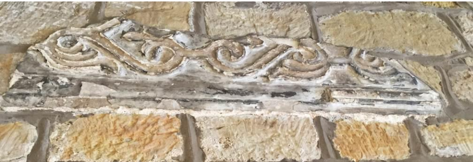
Left: Decorated plasterwork frieze of fleur-de-lis scrollwork above the stone doorway. Courtesy Sara Griffiths
